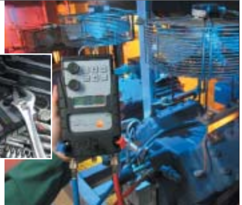
Service and maintenance incl. initial operation of a refrigeration unit
